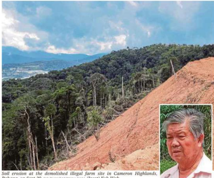
Soil erosion at the demolished illegal farm site in Cameron Highlands, Pahang, on Sept 29. PIC BY NURADZIMMAH DAIM (Inset) Koh Wah.
